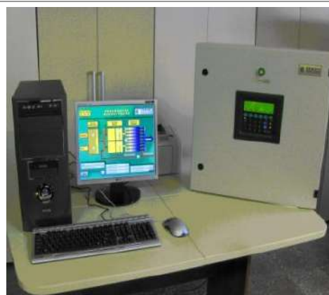
Wastewater Treatment Plant Monitoring and Control
