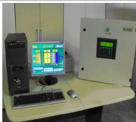
Wastewater Treatment Plant Monitoring and Control
