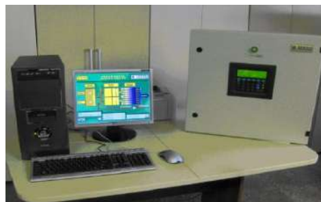
Wastewater Treatment Plant Monitoring and Control
